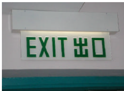
Illuminated exit sign
