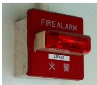
Visual Fire Alarm
