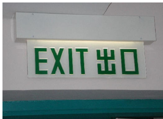
Illuminated exit sign
