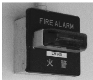
Visual Fire Alarm
