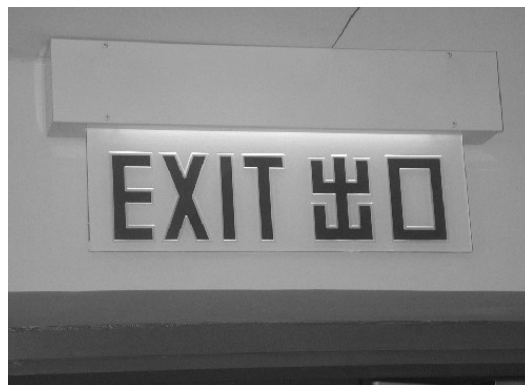
Illuminated exit sign
